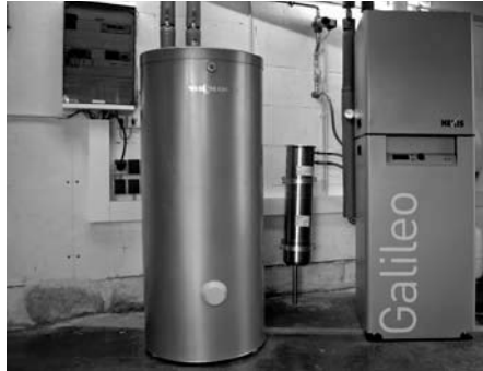
The award-winning fuel cell based combined heat and power unit Galileo 1000 N from Hexis, installed in the basement boiler room of an apartment building.
