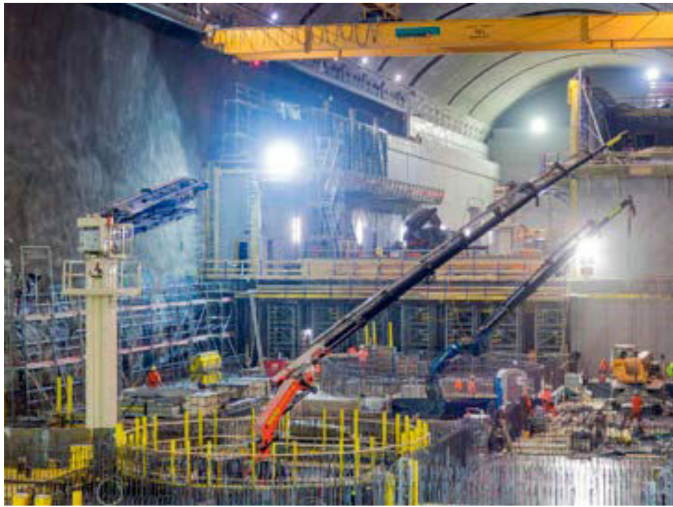
The Nant de Drance pumped storage power station: an epic building project.
