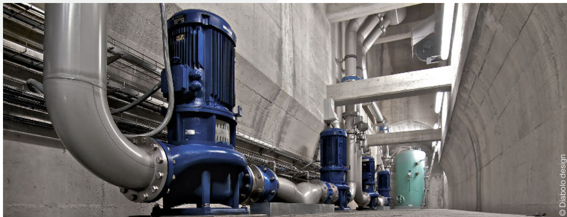
In Vevey, RWB coordinated the rehabilitation of the Les Gonelles water treatment station.
