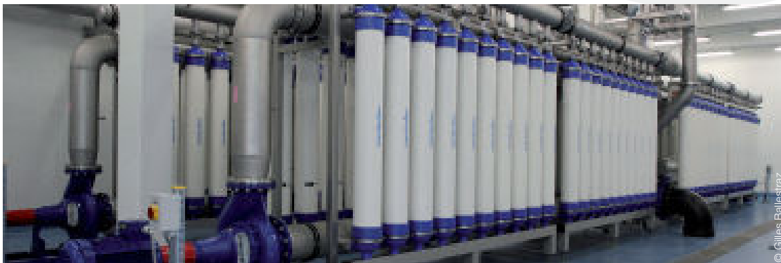
On behalf of the municipalities of Conthey, Ardon and Vétroz, Membrtec has installed an ultrafiltration plant, with a capacity of 500 m 3 /h, for treating water from karstic springs.
