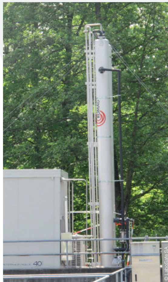
LaboSafe has undertaken a pilot trial in Cham to test the treatment of micropollutants using ozone.
